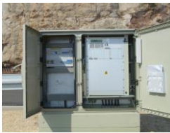
Picture 3: Roadside Outstation independently controls traffic in Local automatic response mode
